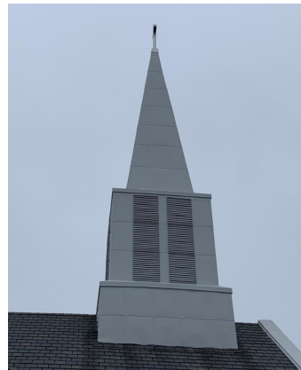
One side of steeple is painted
